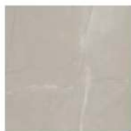
S63069 CA SQUARE Cracked Marble Plaster
